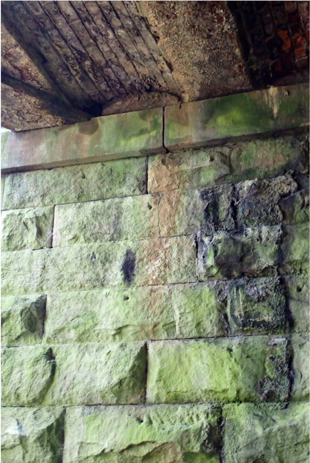
34. Localised crack to a single stone block
