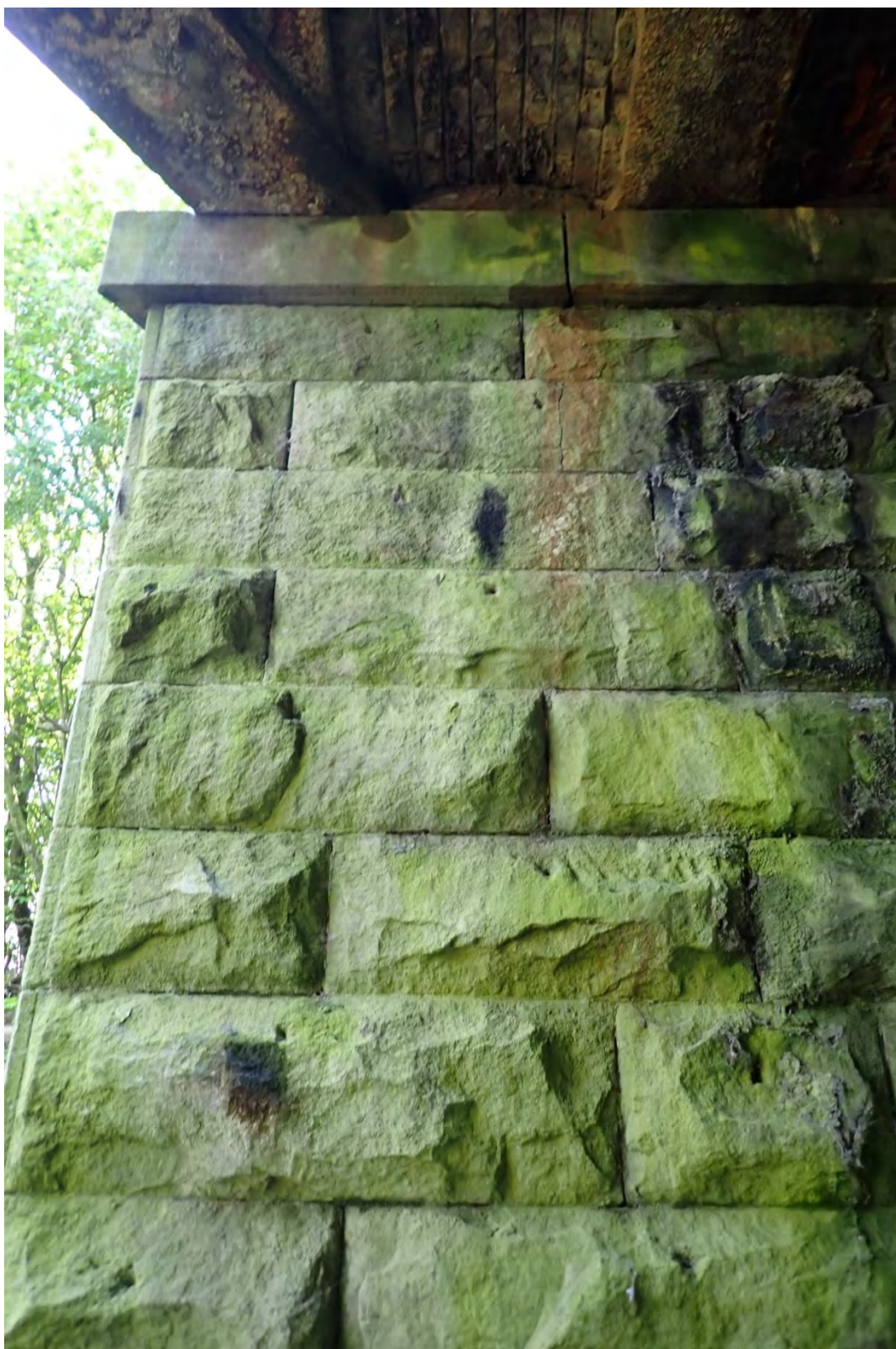
36. SE corner with a localised visible crack to a single stone
