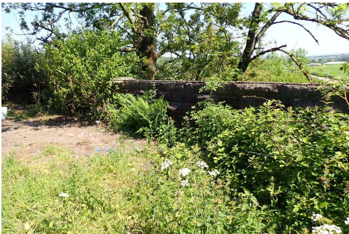
11. South West parapet and overgrown tree and vegetation growth to highway verge
