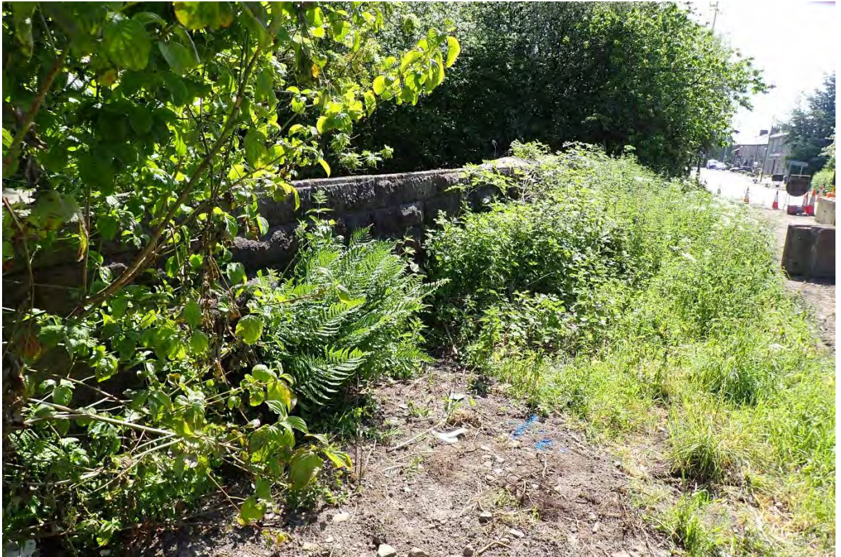
13. North East parapet and tree and vegetation growth along verge
