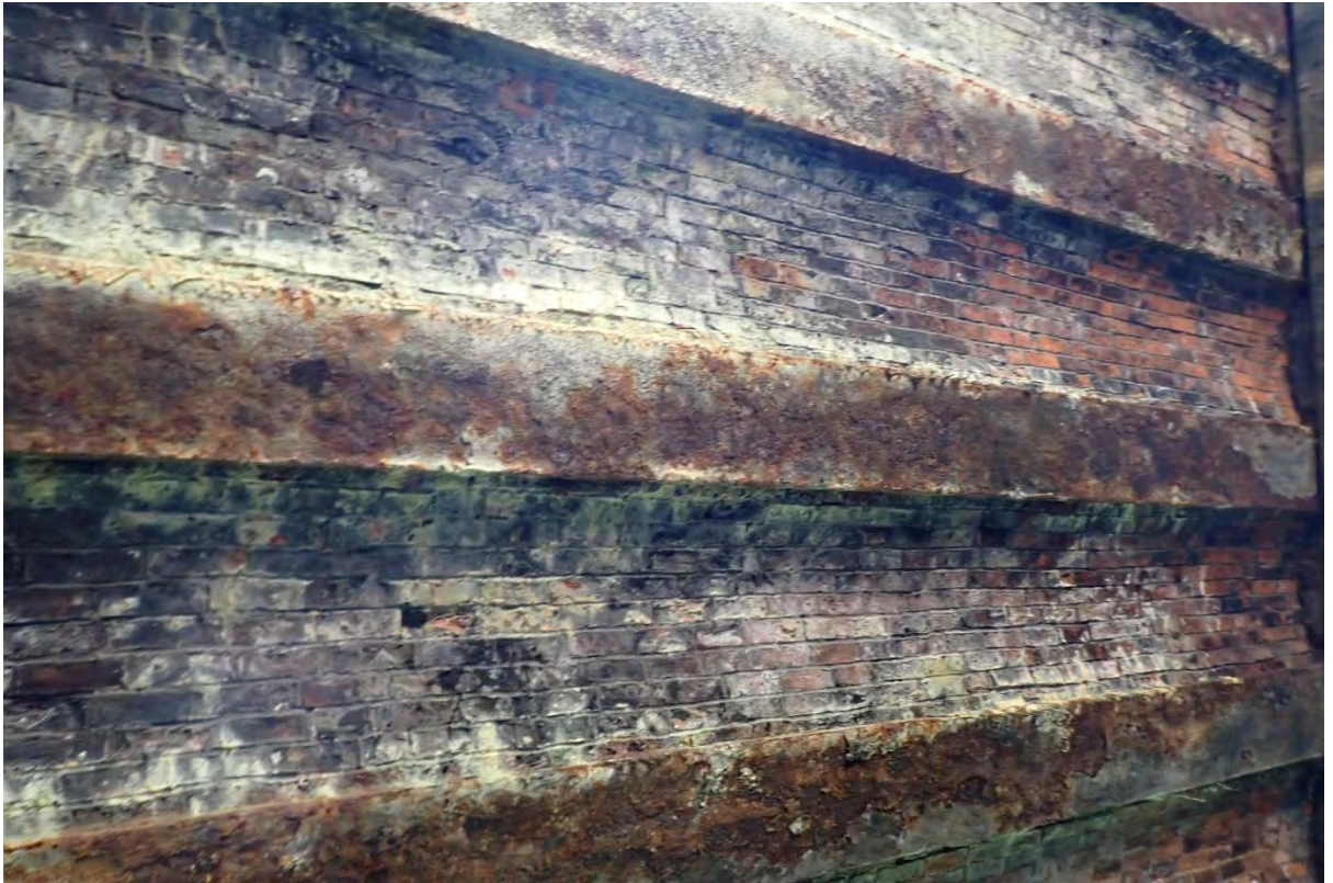
21. Photo showing corrosion to internal deck girders and spalls and mortar loss to brick jack arches
