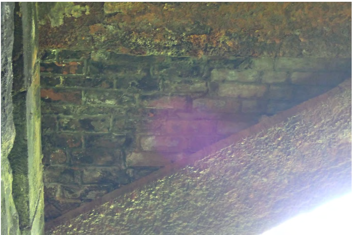
31. Spalls and displacement to the jack arch
