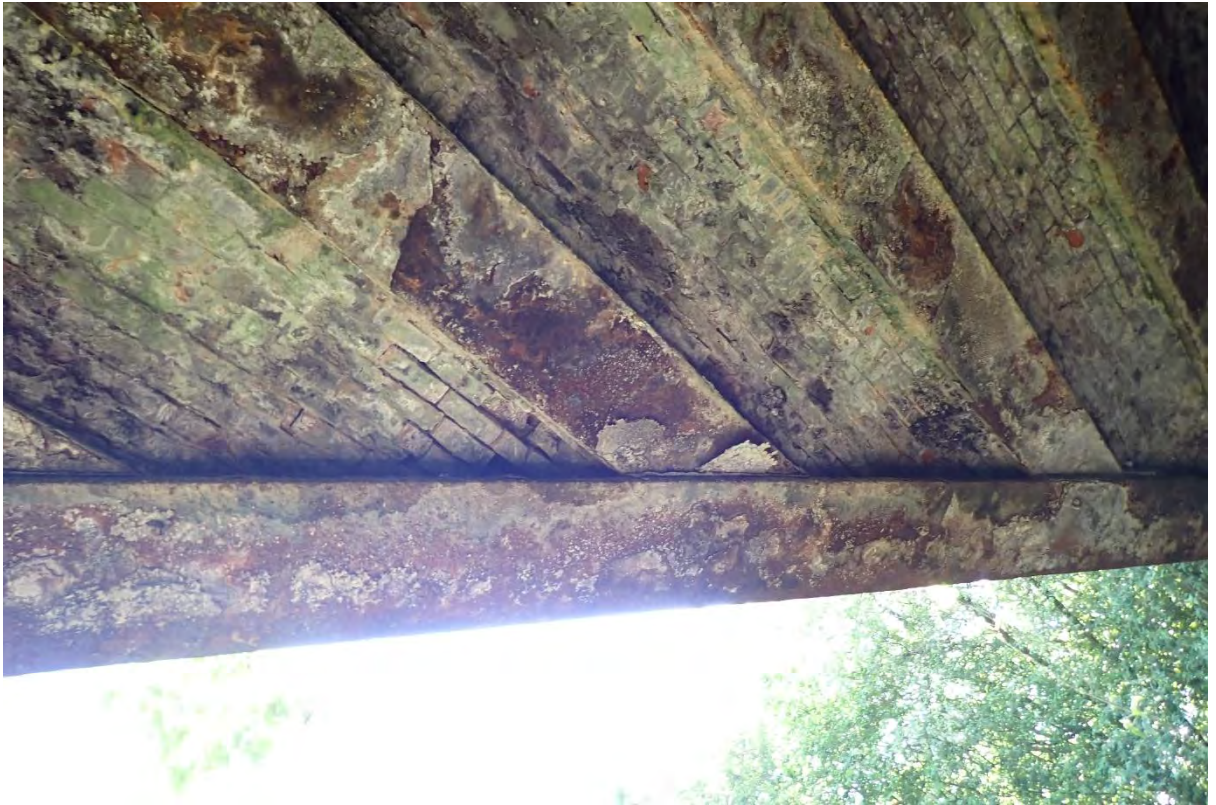
17. Corrosion and delamination to the cast iron beams at the SE end of the bridge
