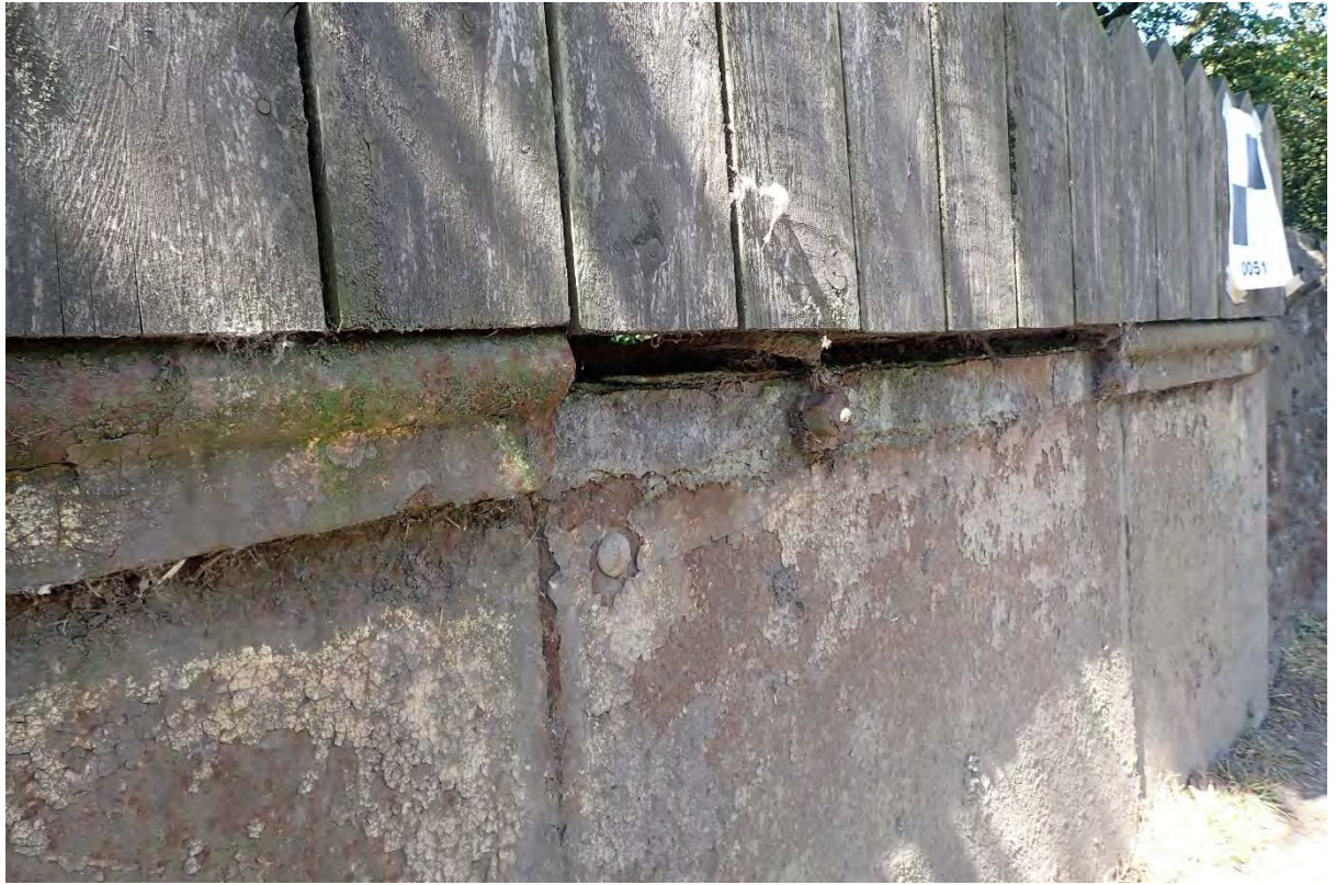
7. Further loss of cast iron section to top of parapet
