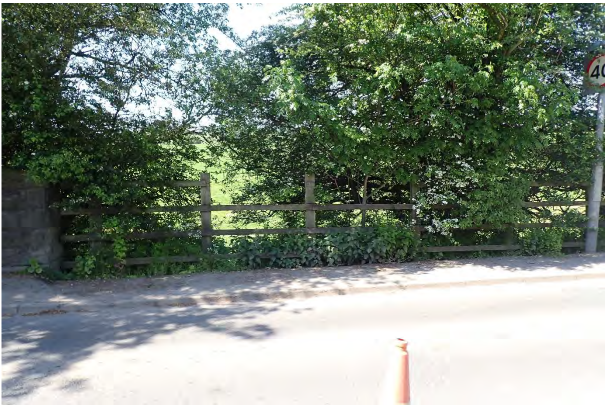
14. Missing timber rails to NW approach fencing
