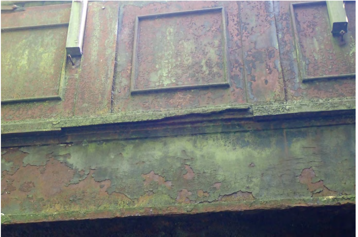
30. Corrosion and section loss to the top flange of the east beam
