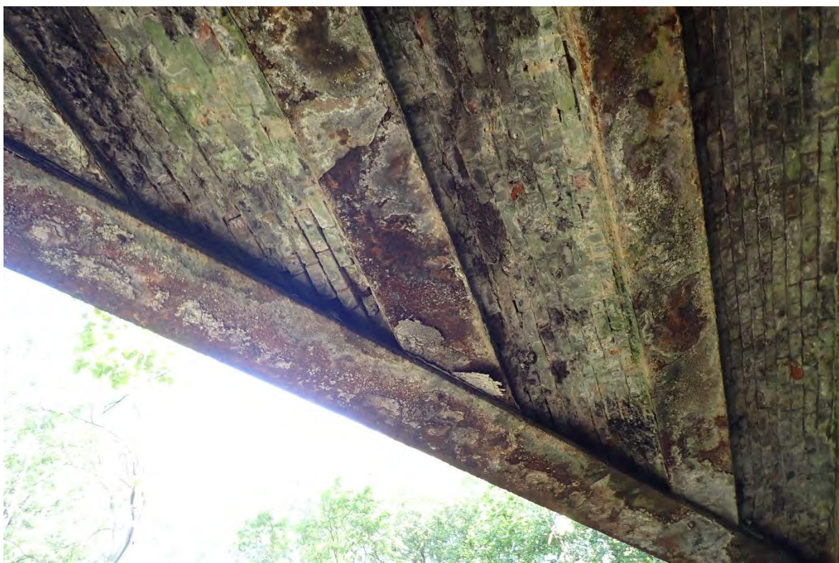
28. External end beam (east) – mortar loss and deformation can be seen to the jack arches
