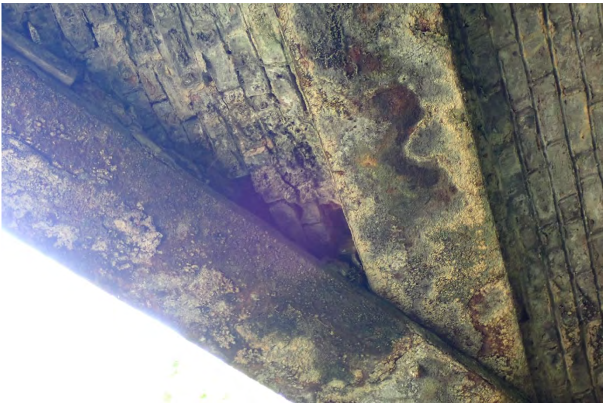
18. Missing bricks to the jack arch due to partial collapse
