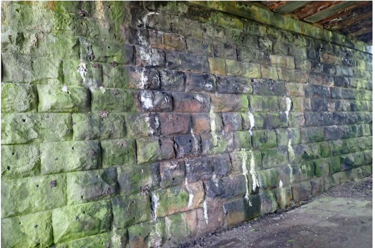
35. Seepage stains to the SE abutment
