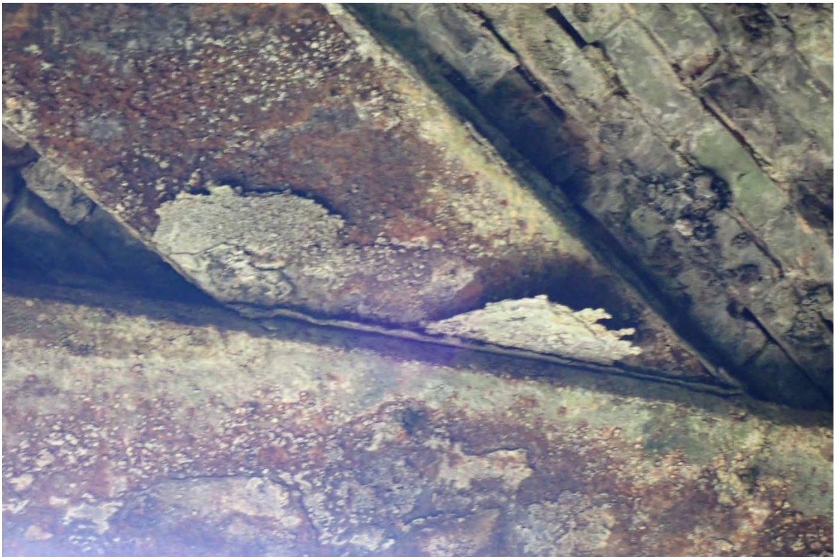
20. Visible delamination, corrosion and pitting to the deck girder along with missing bricks to the jack arch
