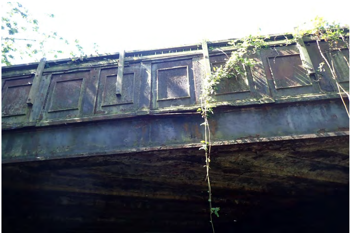
15. View of the rear of the NE parapet and external cast iron beam, with visible corrosion and damage to the top flange
