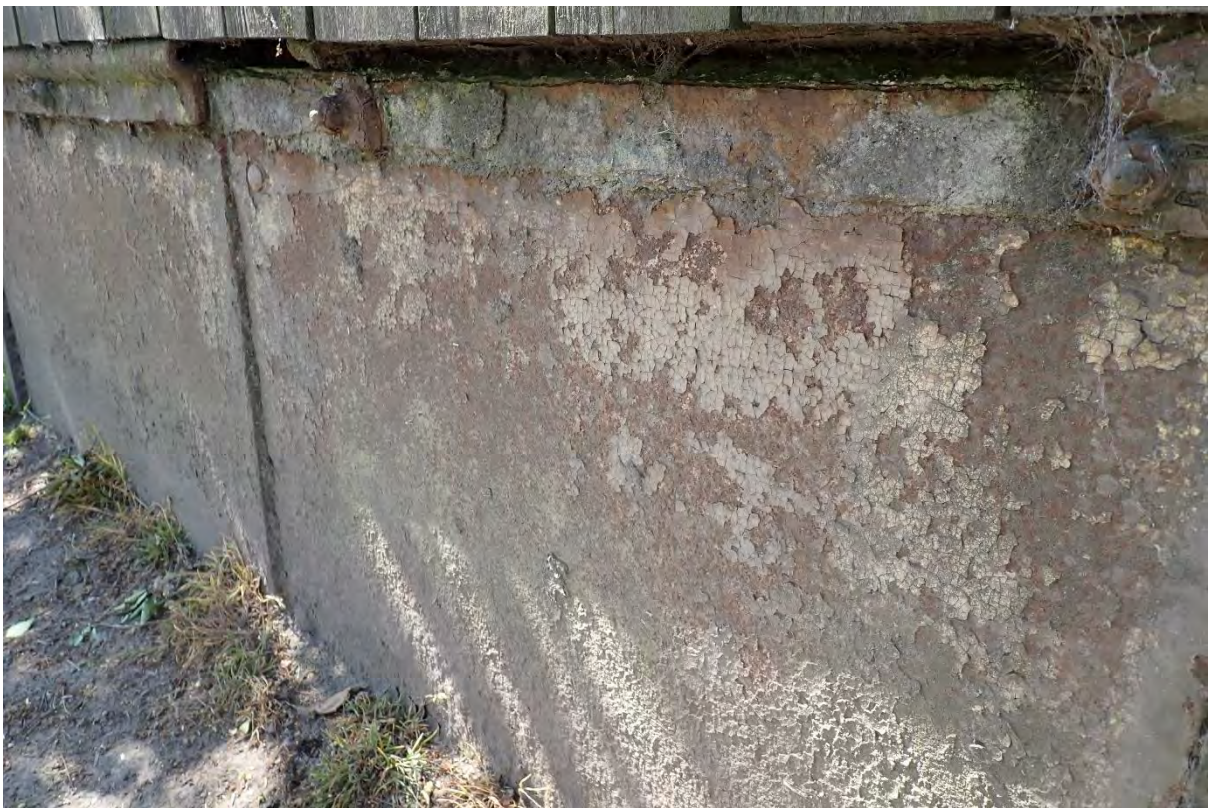
6. Corrosion and loss of cast iron member to the top of the SW parapet
