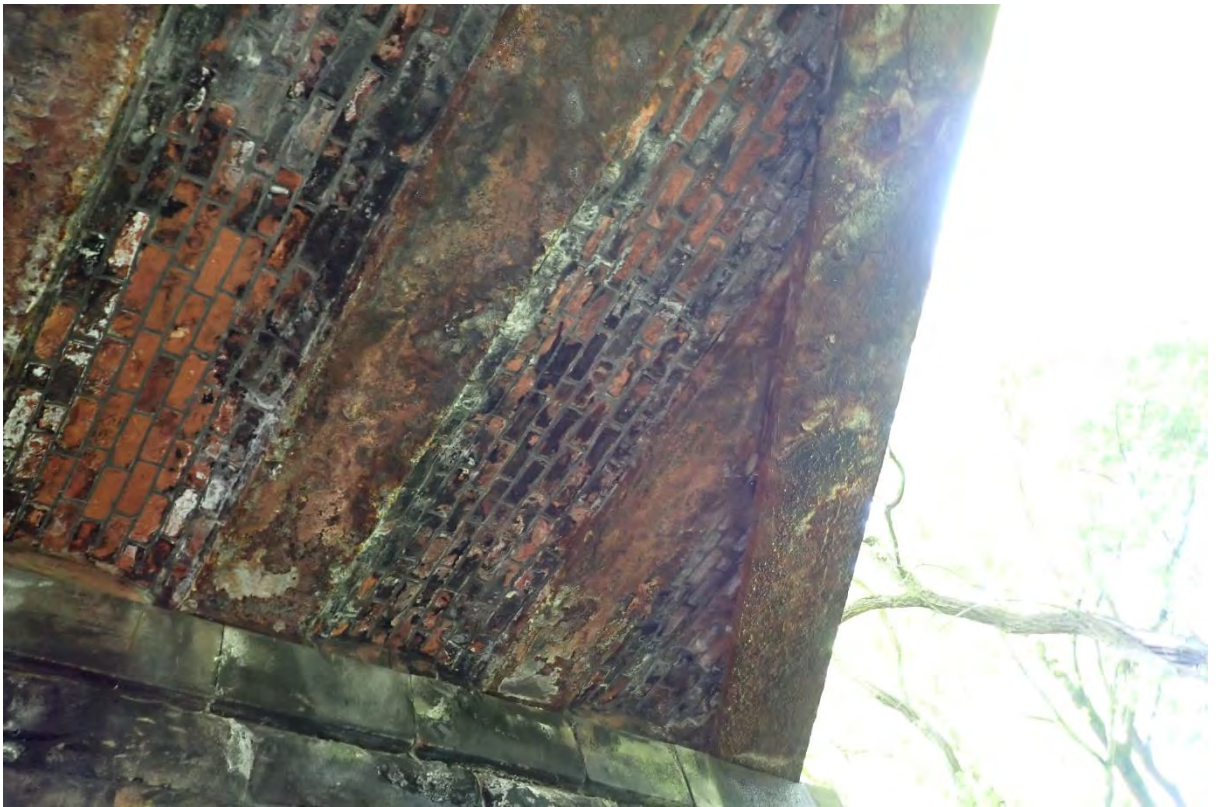
24. SW corner of deck. Visible water drips to external cast iron beam
