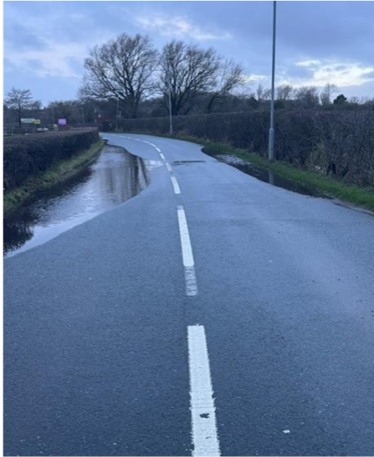
Lancaster Road – surface water from Light rain and over flowing drains
