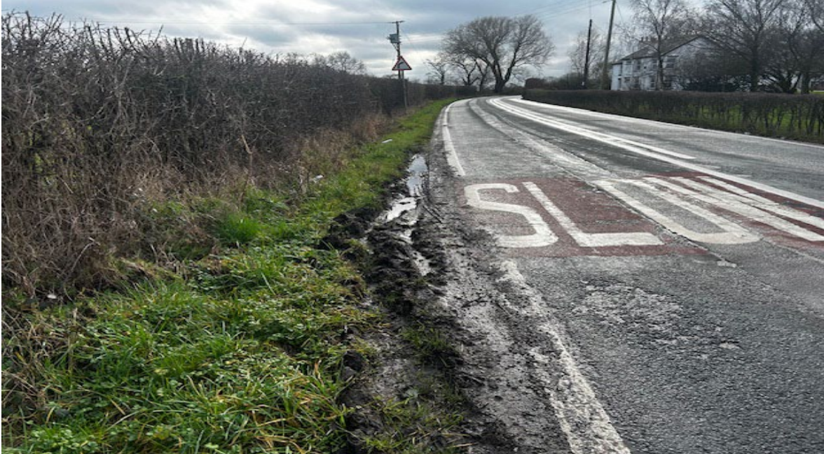
27- Opposite the Access serving Lancaster's Farm access - Verge overrun
