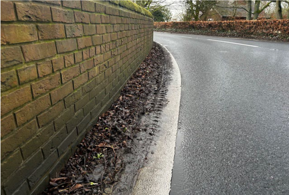
21- Adjacent to the Access serving Fold House Farm - Overrun close to Fold House Farm wall
