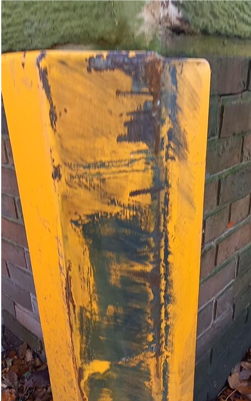
Photograph 2: Damage to the boundary wall at the bend (Image from the site visit conducted on 14 th November 2024).
