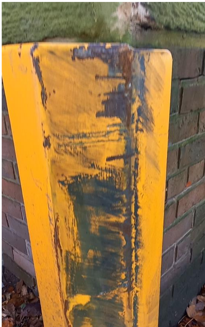
Photograph 2: Damage to the boundary wall at the bend (Image from the site visit conducted on 14 th November 2024).
