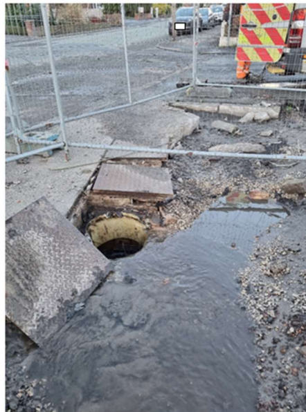
Figure 1 – damage on site in vicinity of culvert collapse
