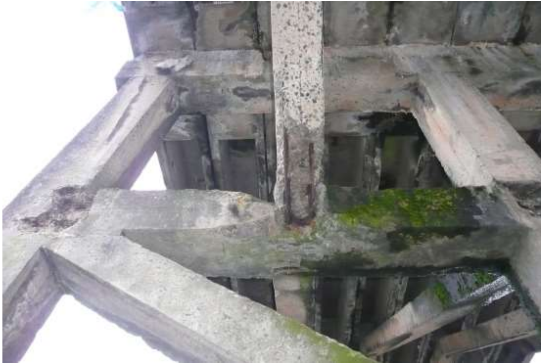
Spalled concrete and exposed reinforcement in the supports with damage from falling struts
