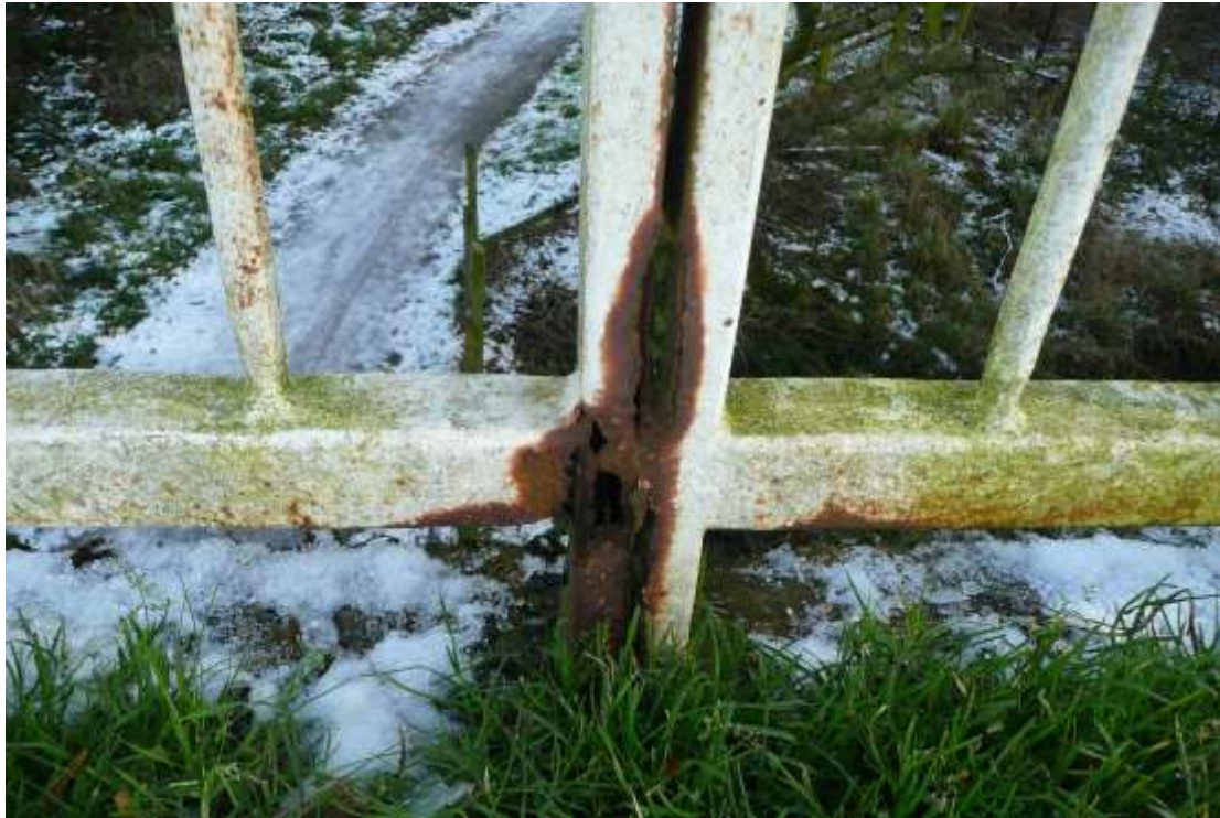
Corrosion of the parapets where they are connected to the bridge
