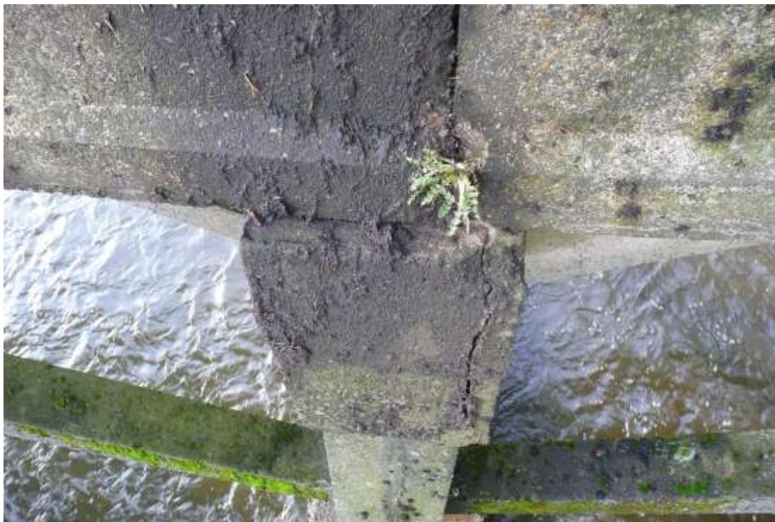
Poor seating of the beams leading to cracking in the support
