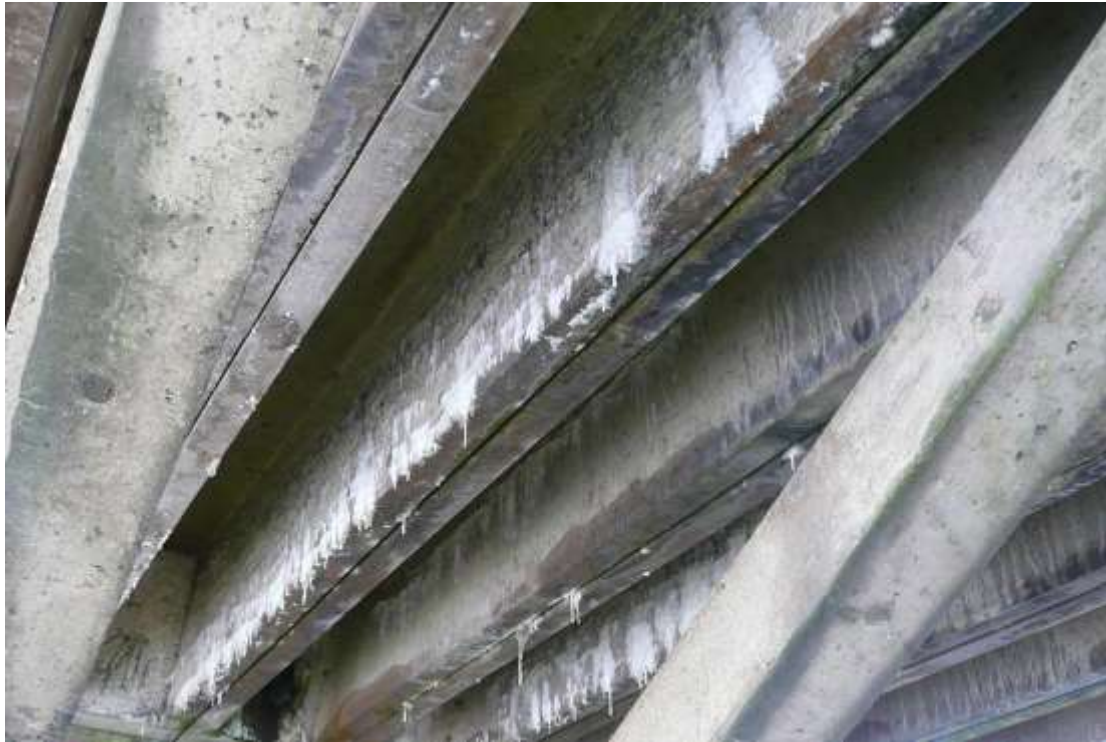
Extensive cracking to the concrete beams with associated leached deposits
