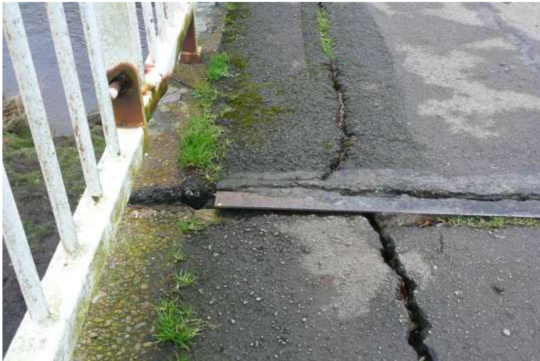
Surface cracking indicating beam movement and allowing water to penetrate the structure
