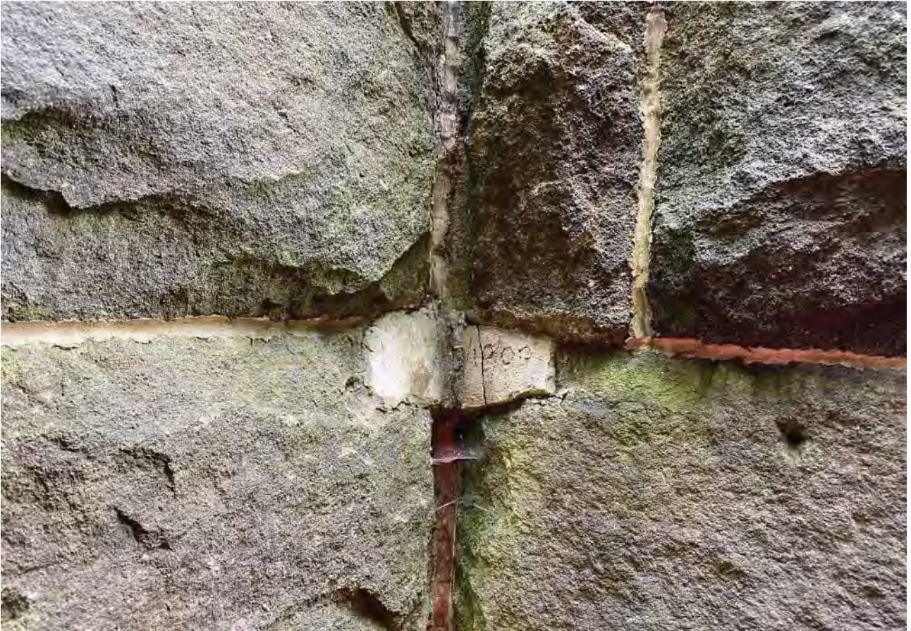
15. Fracture through mortar tab on north east pilaster return
