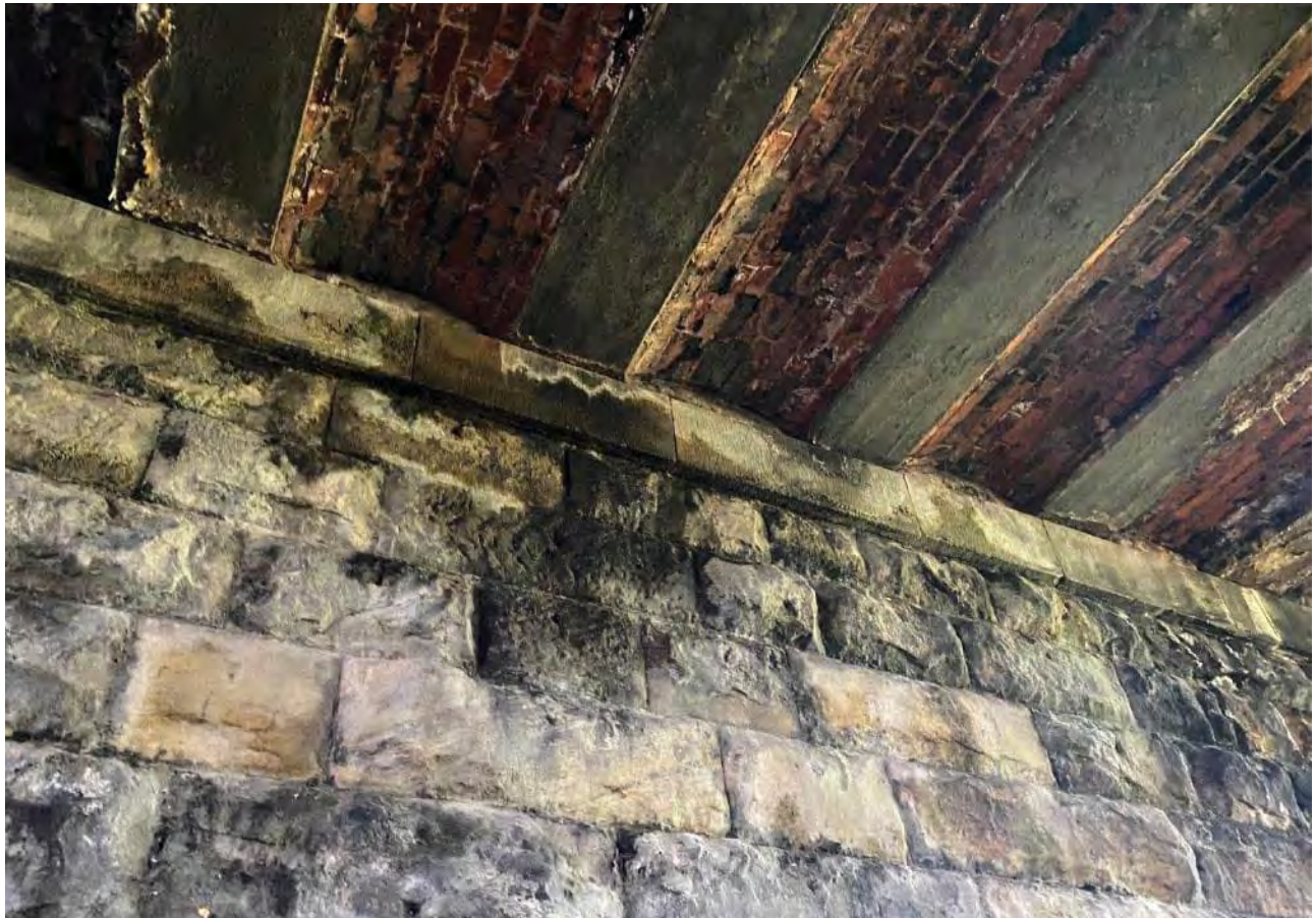
20. Damp on padstones
