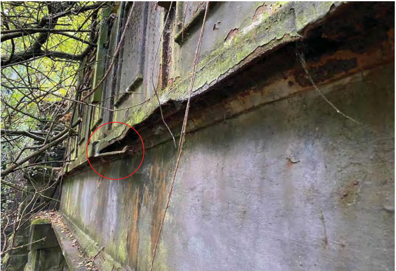
22. Fracture to top flange of edge girder
