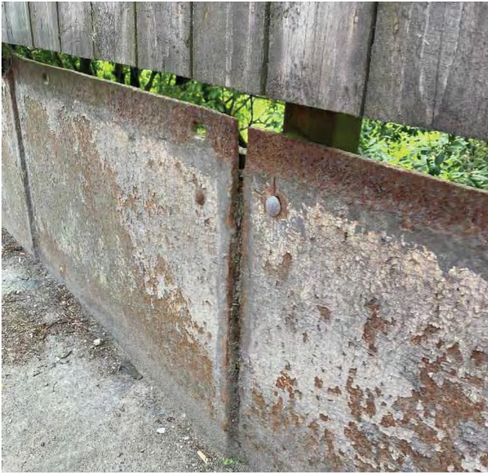
24. Displaced parapet panels
