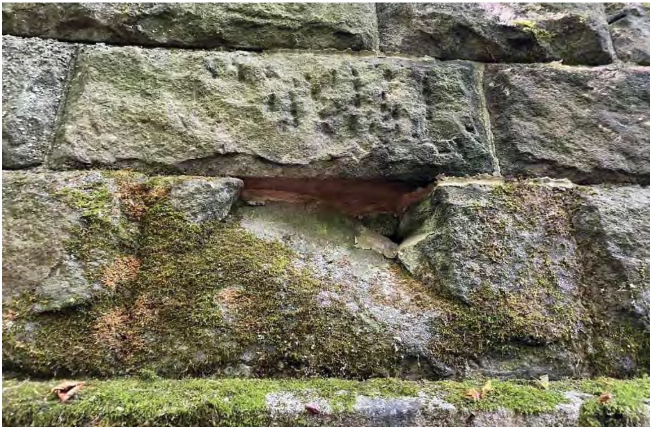
13. Spalling to south east wingwall
