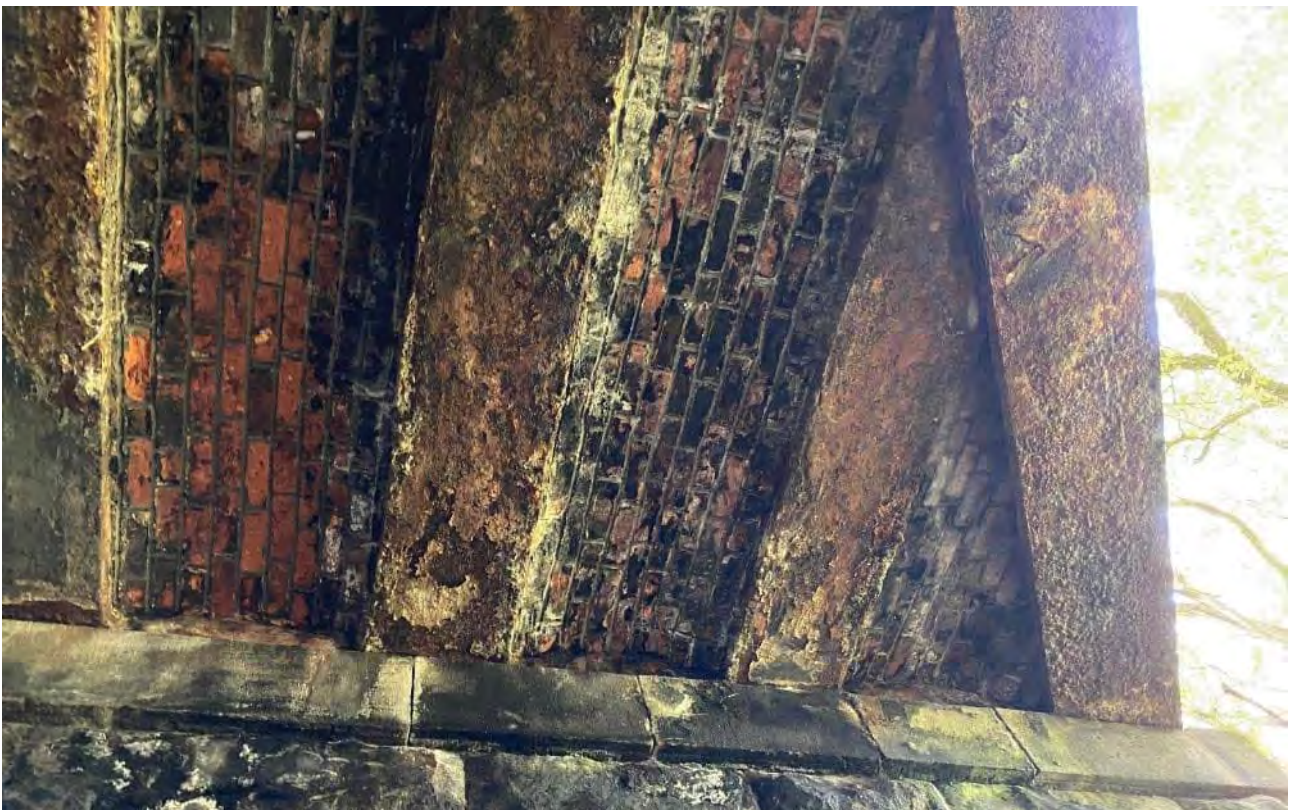
18. Corrosion to edge and internal girders
