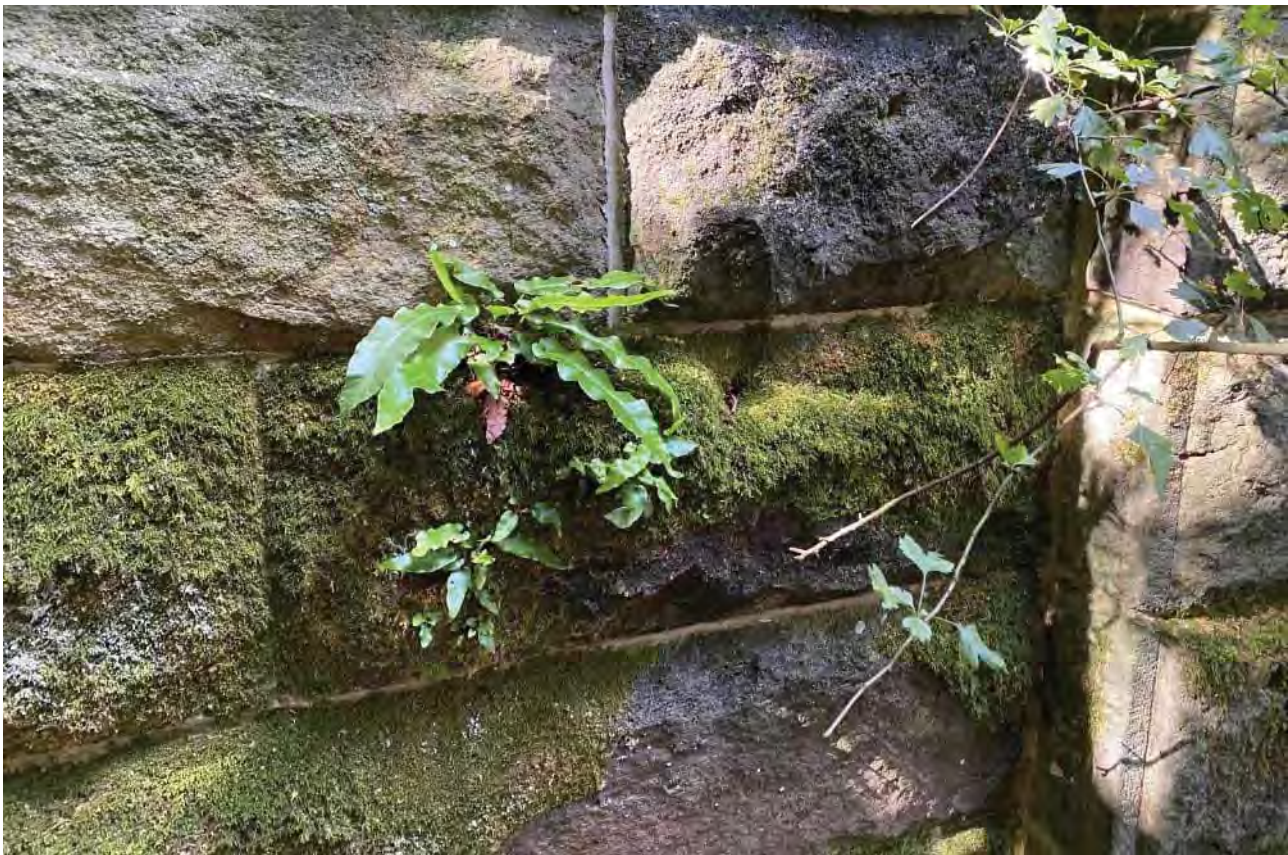
14. Vegetation in joints on south east wingwall
