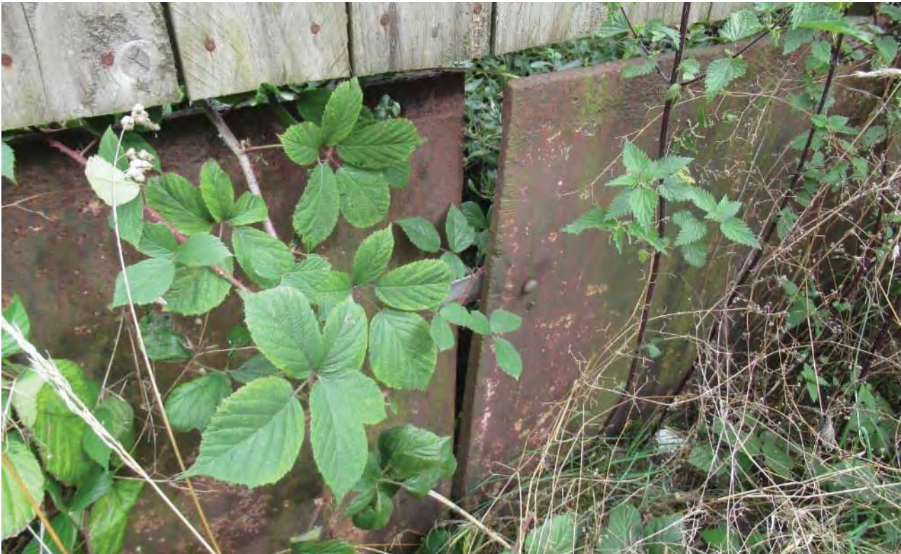
23. Displaced parapet panels
