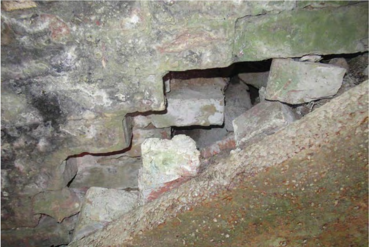
21. Partially collapsed jack arch at north east corner of bridge soffit
