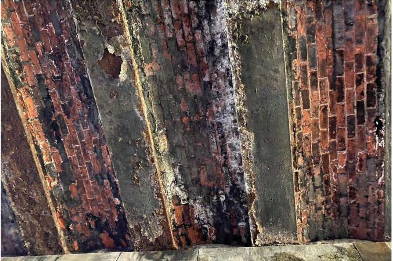
19. Corrosion to internal girders
