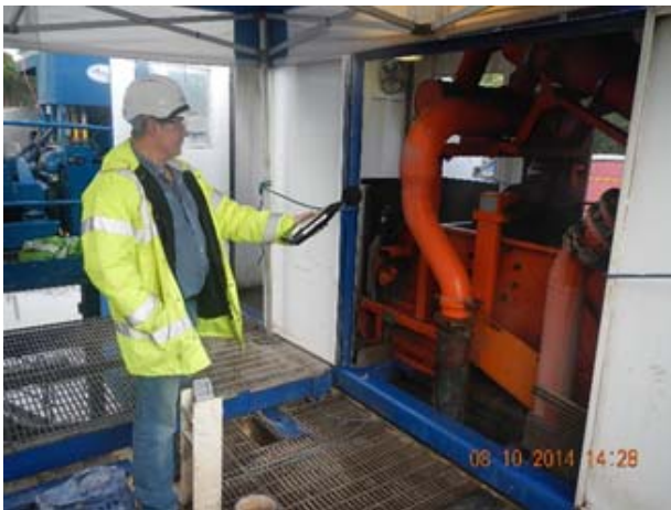
Location 9 – Side on and 1m from Shale Shaker (enclosure hatch open)
