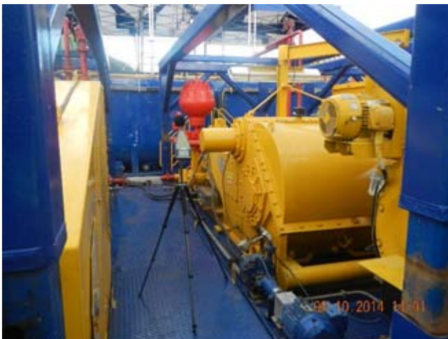
Location 3 - between Mud Pump No.1 and 2, alongside pumps
