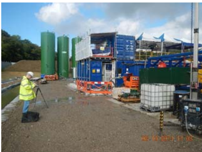
Location 5 – Approximately 9m from Mud Pump No.3 (Mud Pump noise dominant noise source)
