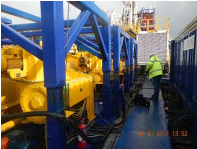
Location 1: 1m from Mud Pump No.2 (electric motor end)
